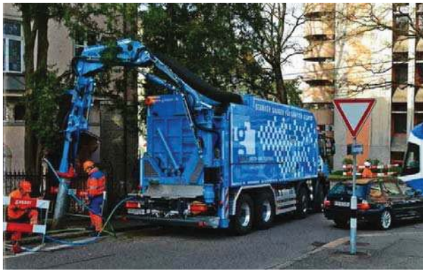
Figure 5. Saugbagger trial to suck in optical cable into duct with power cable
